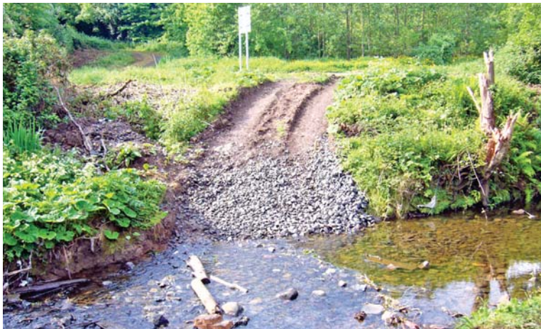
PLATE 15: Bridge Footings 1: bridge footing on south bank of the Three Mile Water.
