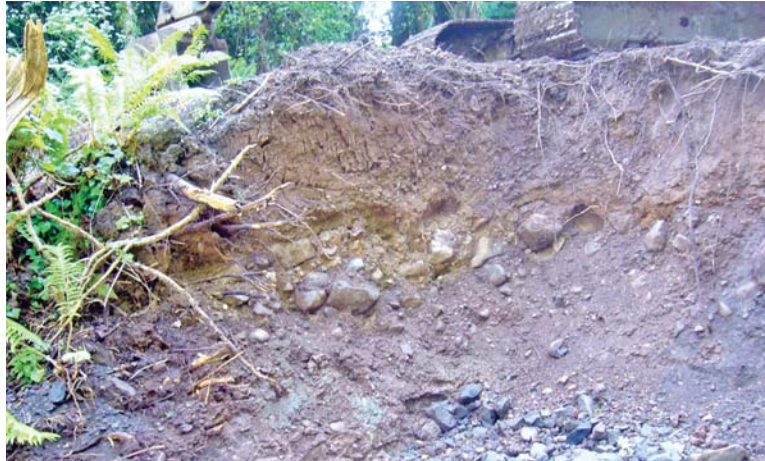
PLATE 22: Bridge Footings 3: detail of bridge footings on southeast bank of Three Mile Water.
