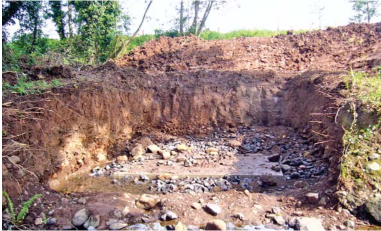
PLATE 19: Bridge Footings 2: bridge footings on north bank of the Three Mile Water.
