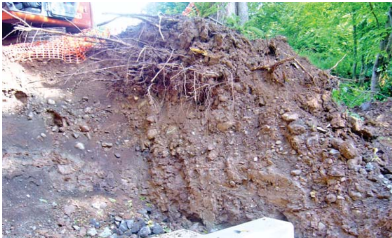
PLATE 21: Bridge Footings 3: detail of bridge footings on northwest bank of Three Mile Water.
