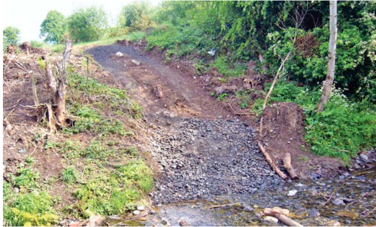
PLATE 16: Bridge Footings 1: bridge footing on north bank of the Three Mile Water.
