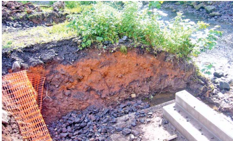
PLATE 23: Bridge Footings 4: the southwest facing section of bridge footing on north bank of Three Mile Water.
