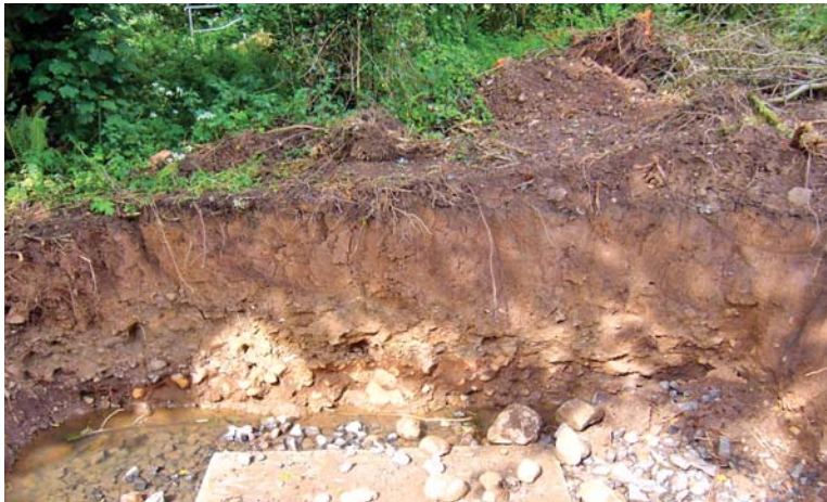
PLATE 20: Bridge Footings 2: detail of east facing section of bridge footing on north bank of the Three Mile Water.
