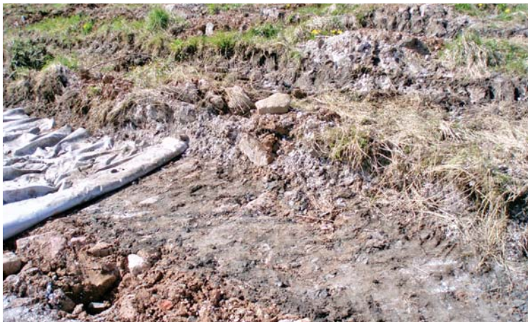
PLATE 8: Section 2: detail of partially constructed footpath showing depth of excavation into imported hardcore surface.
